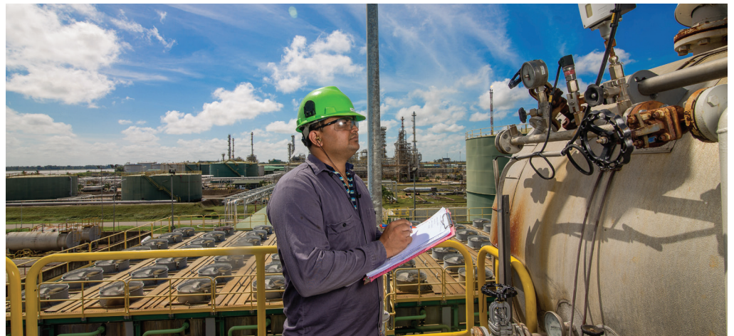
An employee of SPCS (Staatsolie thermal plant) at work with the refinery as background
